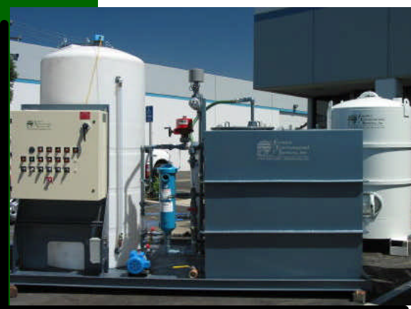
Front: 10 GPM Vacuum Air Stripper Back: 2000# Carbon Adsorption Vessel
