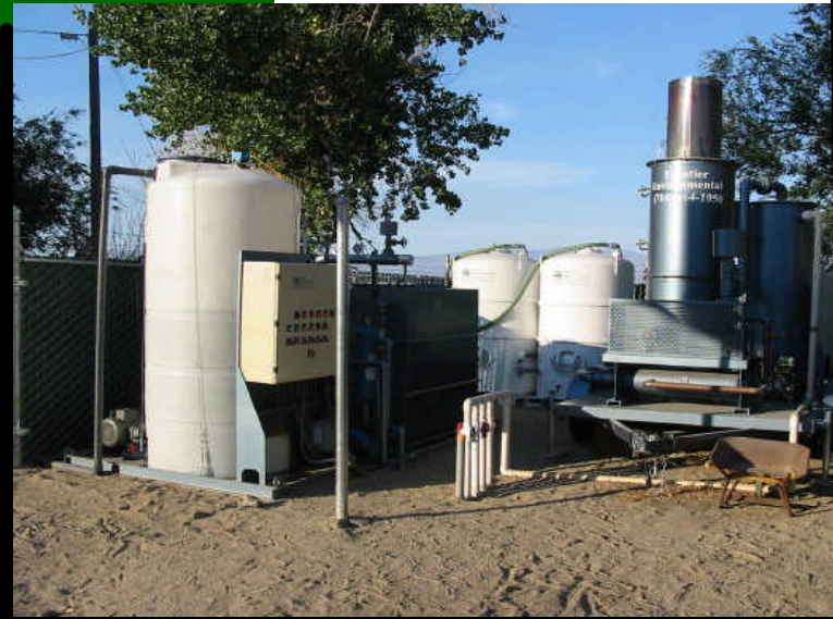
Operational 250 CFM Thermal Oxidizer w/ Water Treatment
