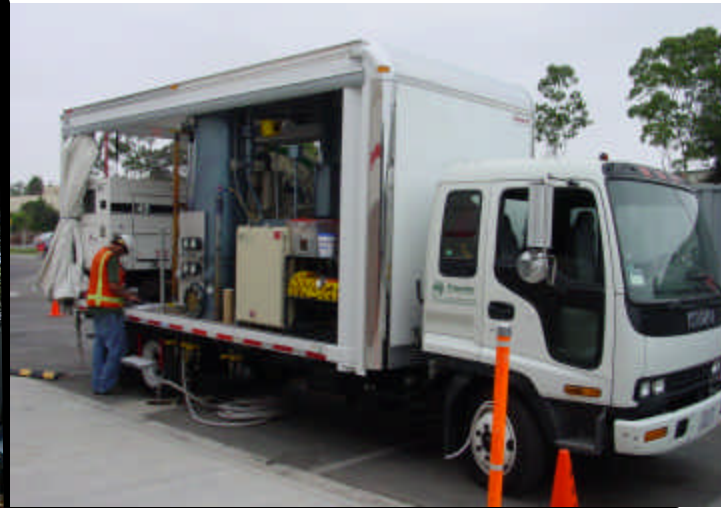
Self Contained Mobile Treatment / Pilot Study System w/ 420 ACFM Thermal oxidizer, Electrical Generator, And Operator
