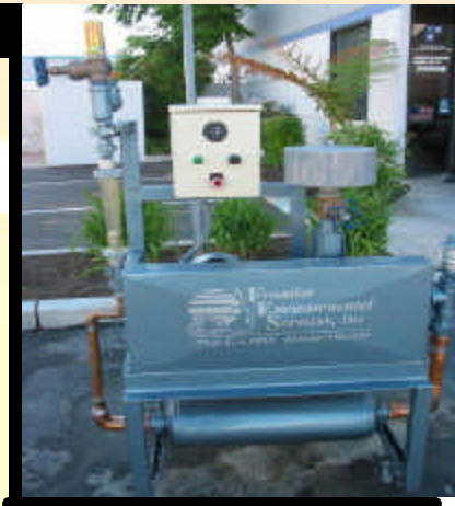
100 CFM Air Spurge w/ Positive Displacement Pump
