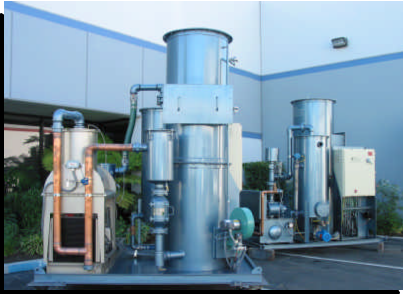
Front: 450 ACFM Thermal/Catalytic Oxidizer w/ Oil Sealed Liquid Ring Pump Back: 250 SCFM Thermal/Catalytic Oxidizer w/ PD Pump
